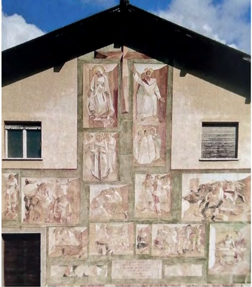
The fresco on the western facade of the former "social house" of Godenzo, before and after the restoration
